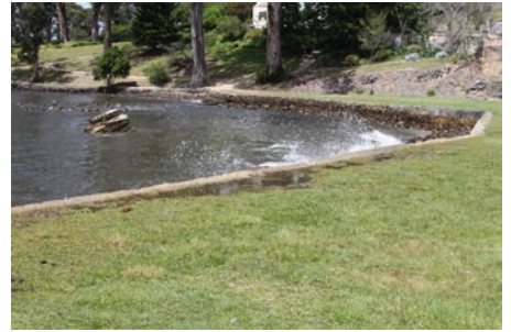
PHOTOGRAPH 2-26 MASON COVE SEAWALL ADJACENT TO PENITENTIARY – HIGH TIDE WATER ACTIVITY
